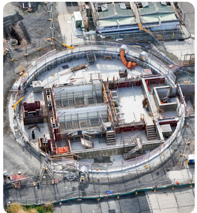
New pump station at Macquarie Point
