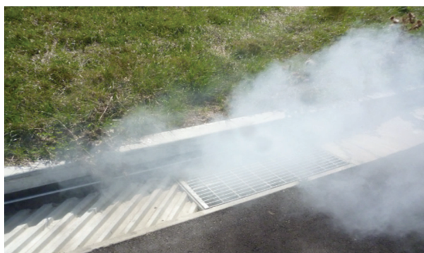
The photo above shows vapour escaping from an incorrectly connected council stormwater pit.
